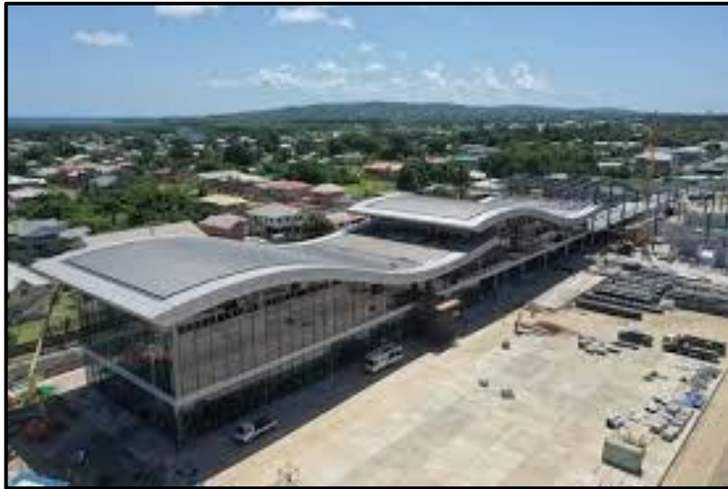
New Terminal in TAB, Tobago where consideration being considered for duty free shopping and shopping for cruise ship passengers
