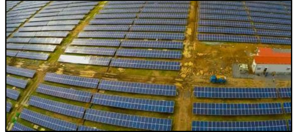
Above, 45 acre solar park at Cochin Airport, India
